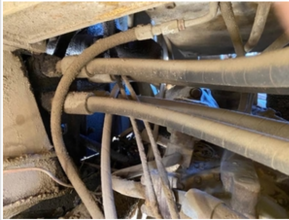
Appearance of Hydraulic Lines / Fittings Photos
