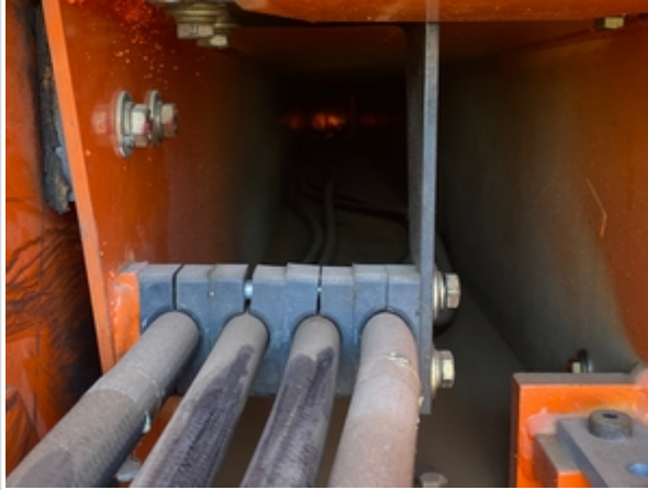
Appearance of Hydraulic Lines / Fittings Photos
