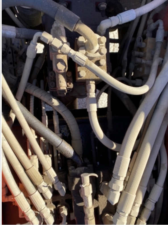
Appearance of Hydraulic Lines / Fittings Photos
