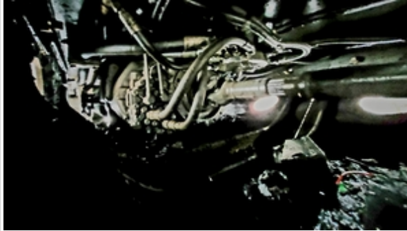
Hydrostatics Pump main area, beneath center of machine has minor oil buildup on surface of bottom machine guards.
