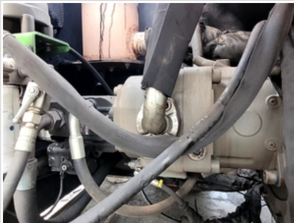
Main hydraulic pump
