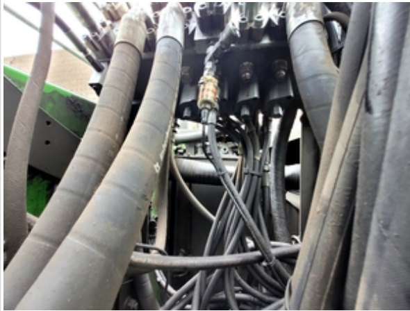
Bottom of Main control valve
