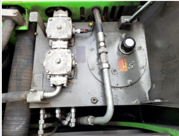
Topside of Hydraulic Tank
