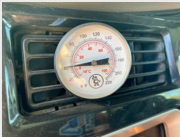
A/C functioning well
