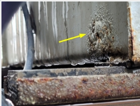
Rust on front lower side of water tank (Behind left side of Cab)
