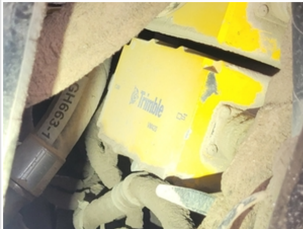
Trimble control unit installed (Not Tested)
