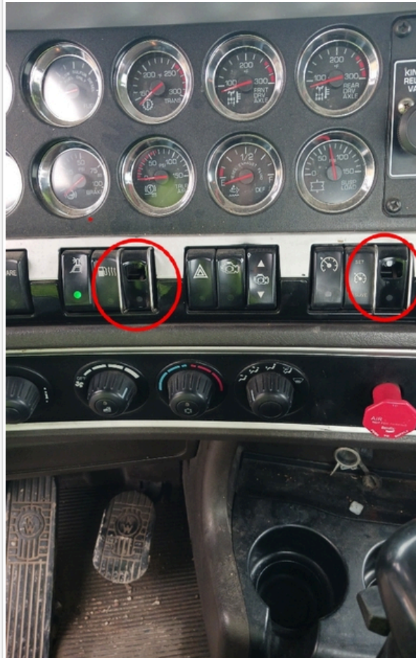
2 switches are missing small covers for switches
