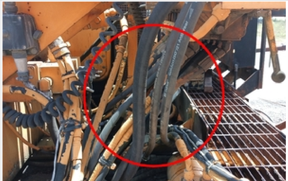
hoses have above normal wear and tear
