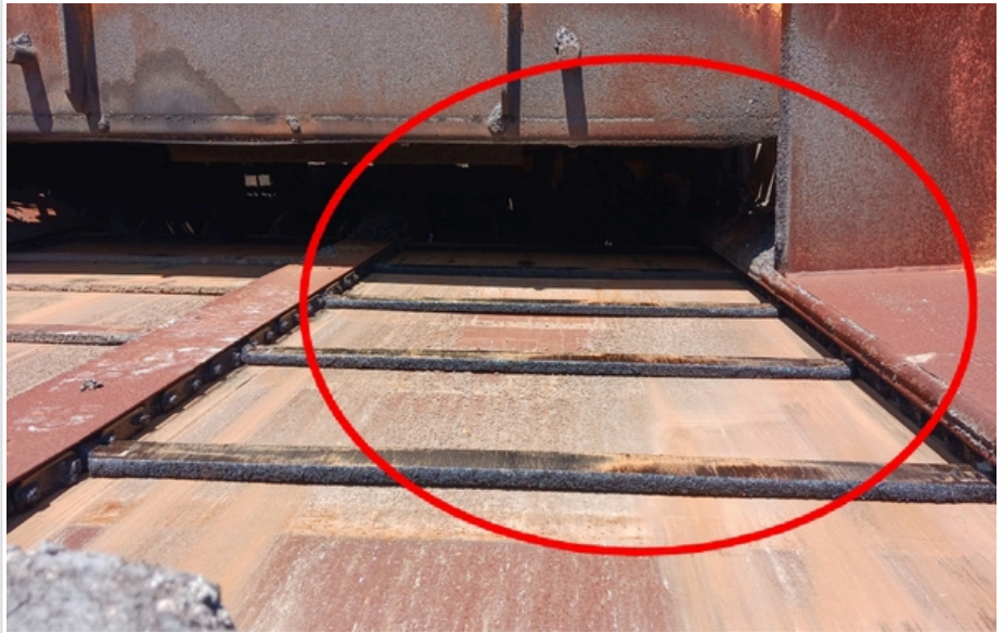
left side of hopper has rust
