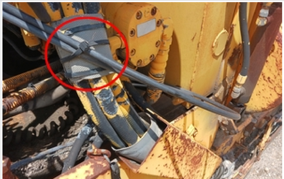
zip ties on hoses
