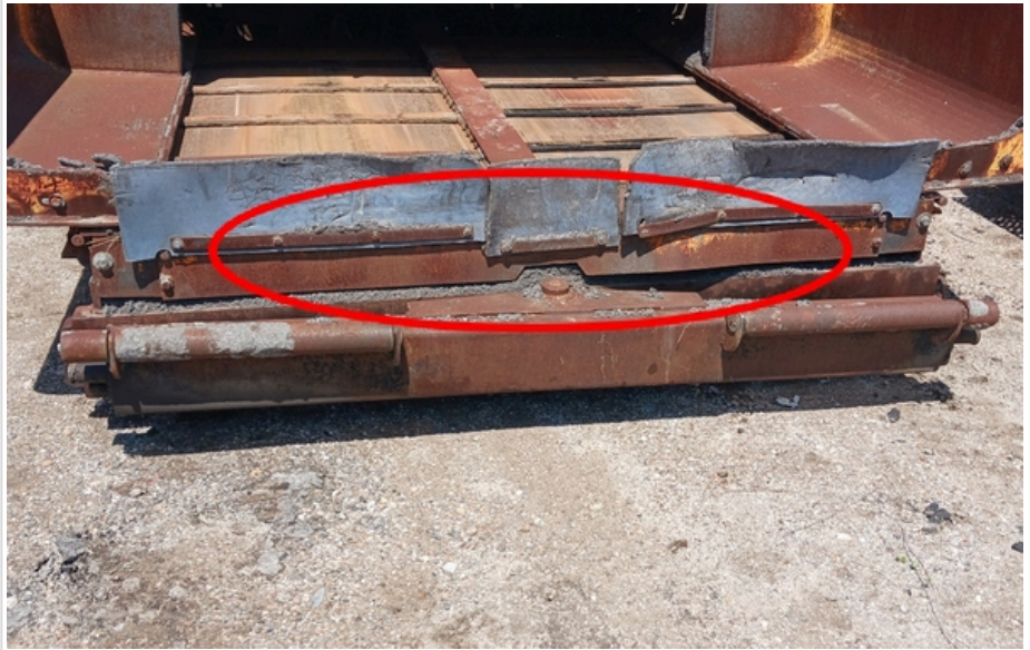
flashing front strips are bent/warped
