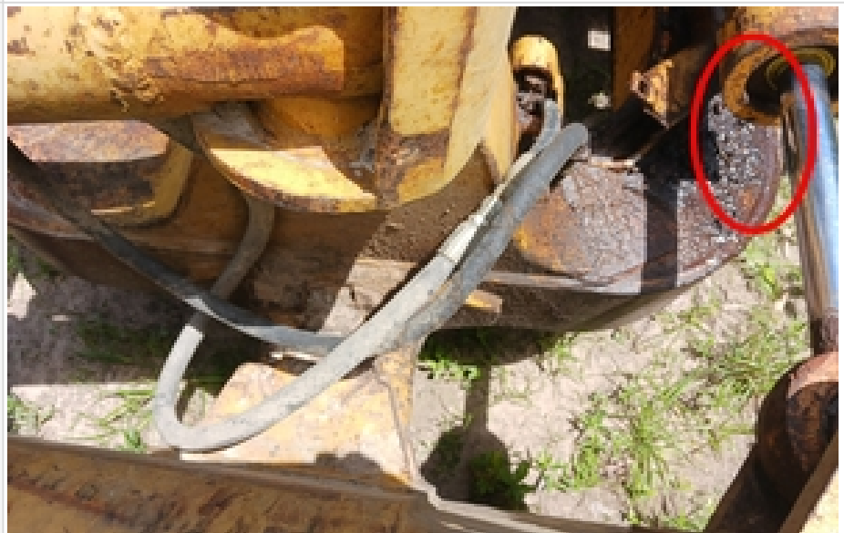
leak from under hose guard on left hand side arm cylinder
