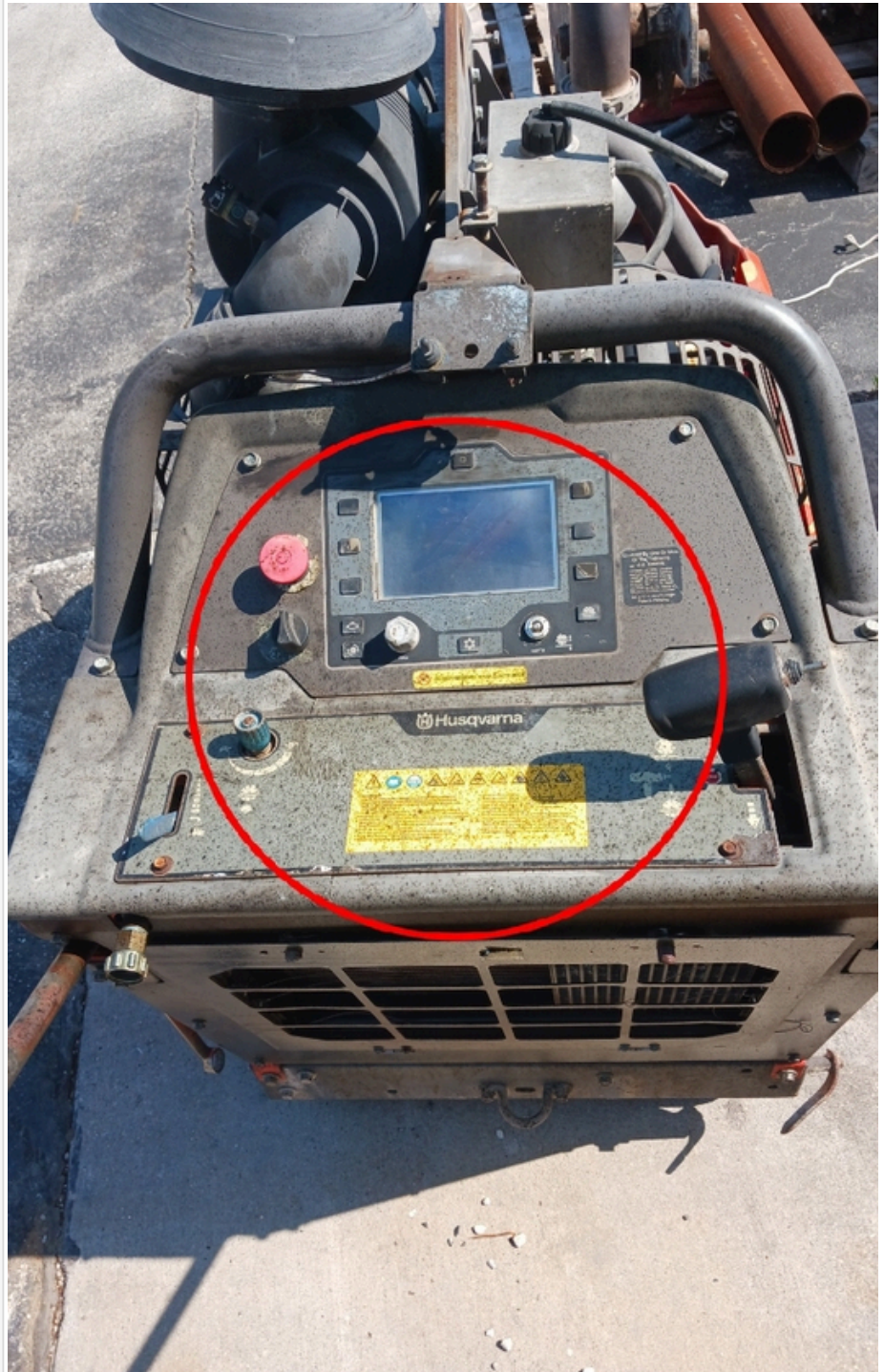
station is dirty
