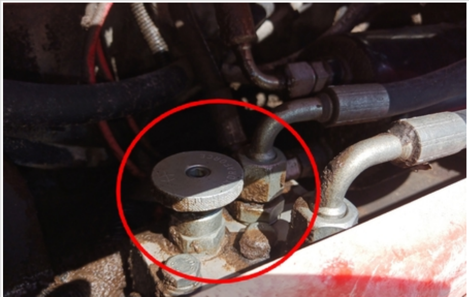
area is wet, signs of a small leak
