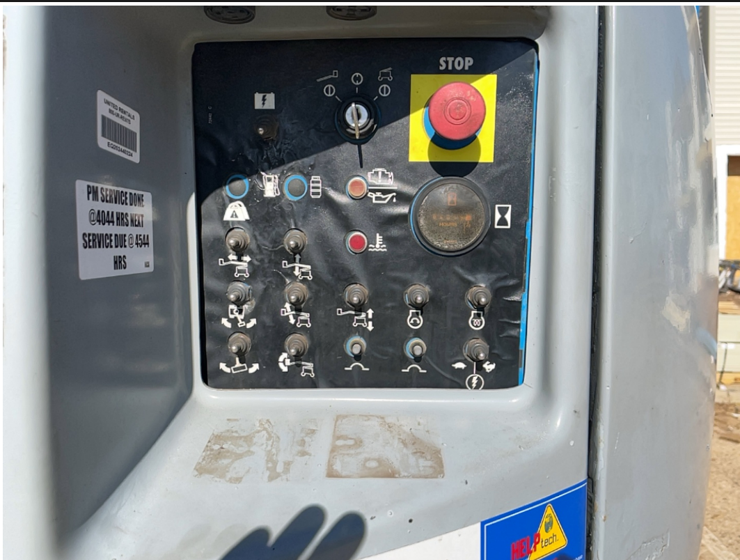
Switches and Controls / EMS Warning Lights / 02-26-2024
