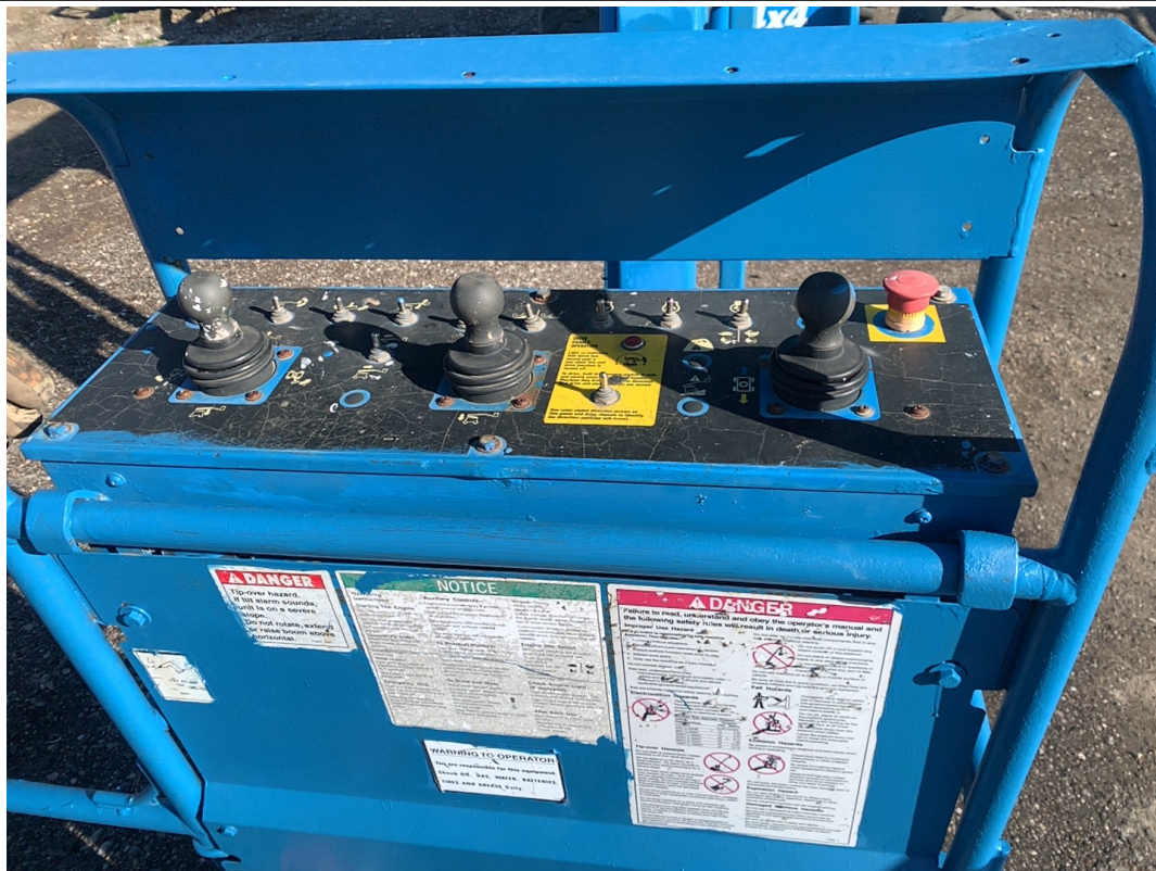
Switches and Controls / 03-27-2024
