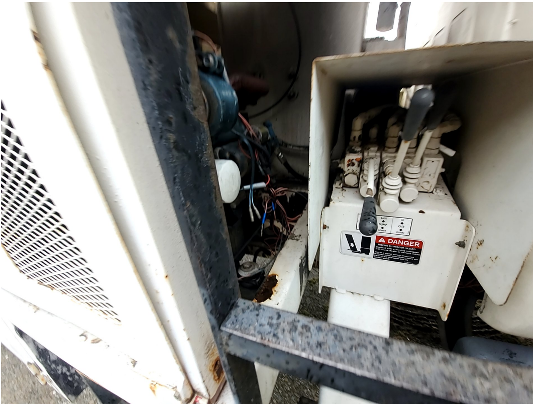
Switches and Controls / 04-04-2024
