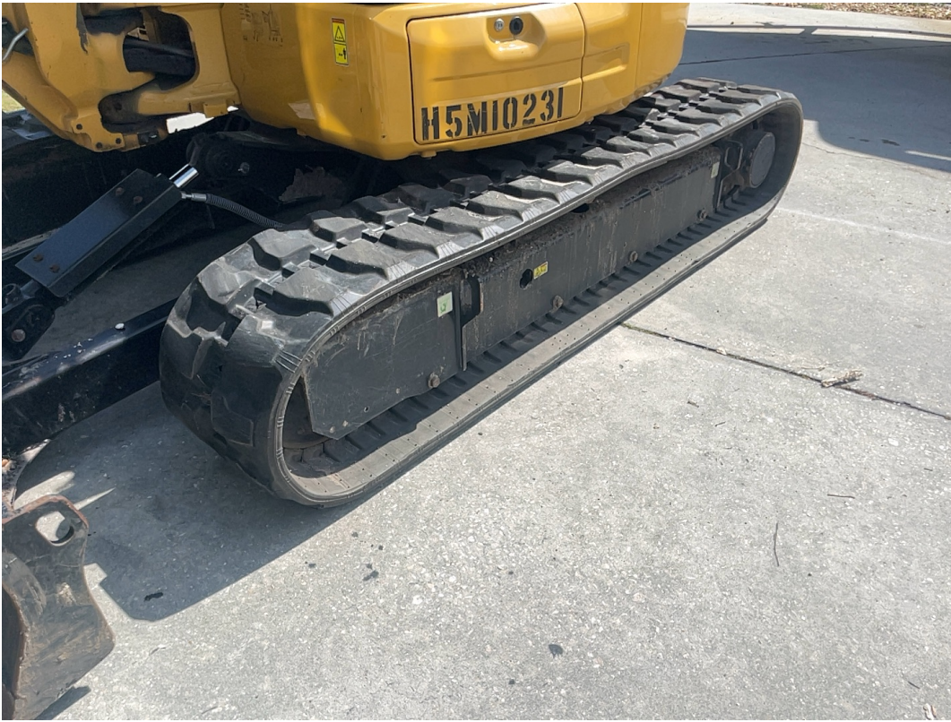
Left Track Condition / 04-04-2024
