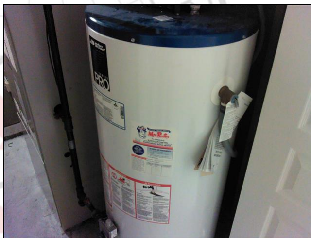
Hot water tank age
