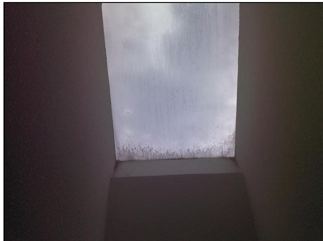
Broken skylight seals
