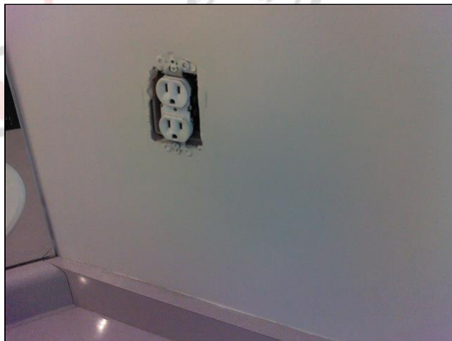
Missing outlet cover
