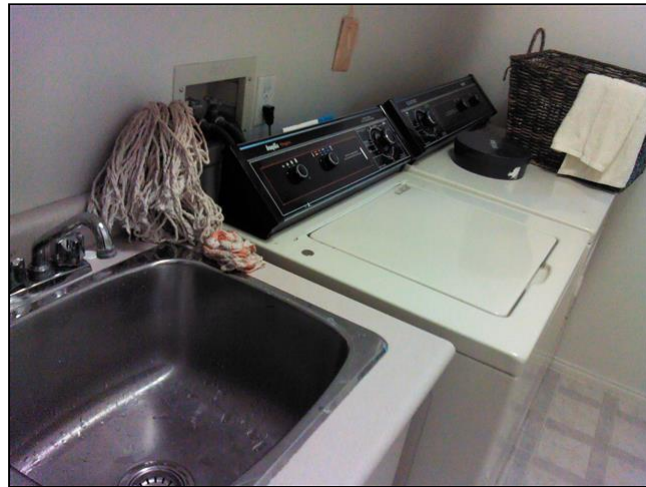
Dryer vent disconnected
