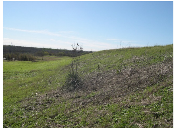
Figure 8: Bush on Downstream Embankment
