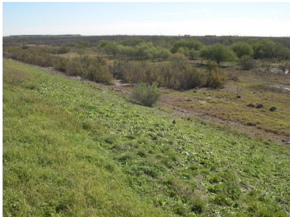
Figure 7: Tree on Downstream Embankment
