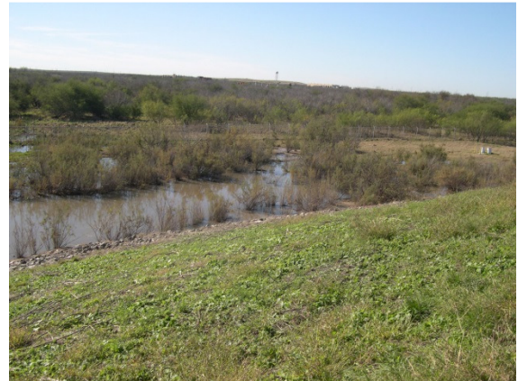
Figure 10: Ponded Water Toe of Embankment
