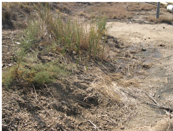
Figure 19: Toe Seep on Downstream Embankment
