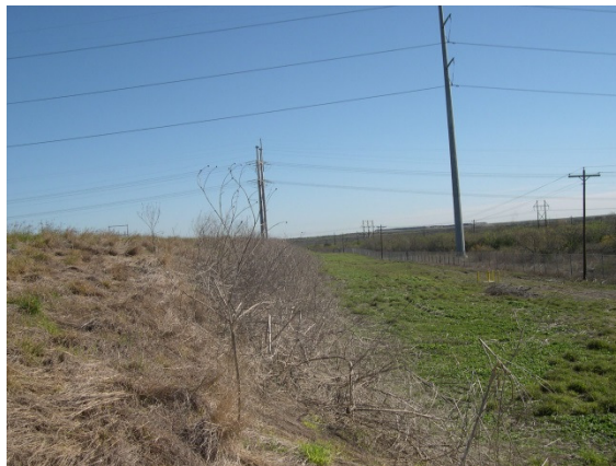
Figure 17: Tree/Bush on Downstream Embankment
