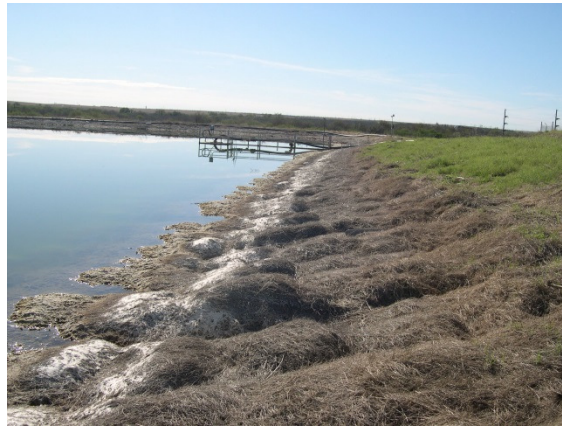
Figure 3: Wind/Wave Erosion Gullies
