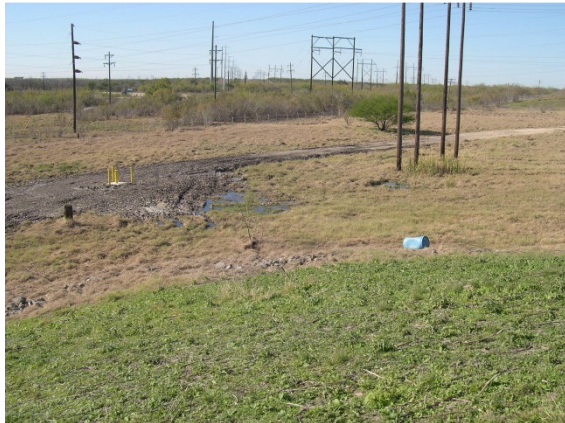
Figure 9: Ponded Water Toe of Embankment
