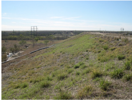
Figure 18: Ponded Water Toe of Embankment
