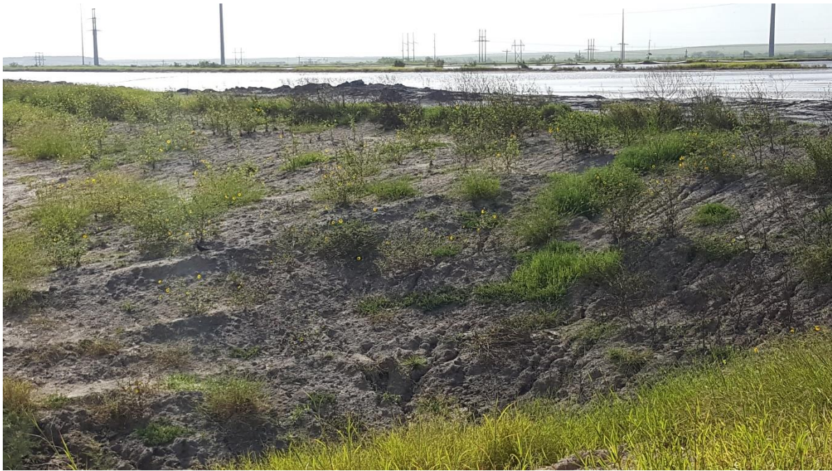
Photo 1 – View looking southeast of west end of north downstream slope of Ash Water Transport Pond.
