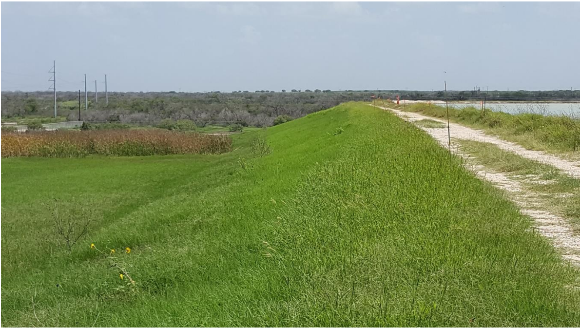
Photo 16 – View looking east from near northwest corner of pond at north embankment.
