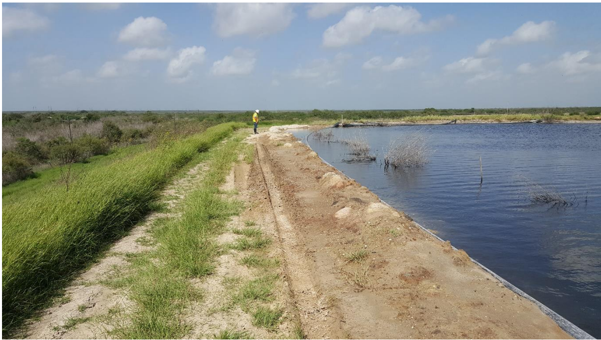
Photo 7 – View looking west at south slope where there is rutting at crest, temporary berm due to high water level in pond and bushes on upstream slope.
