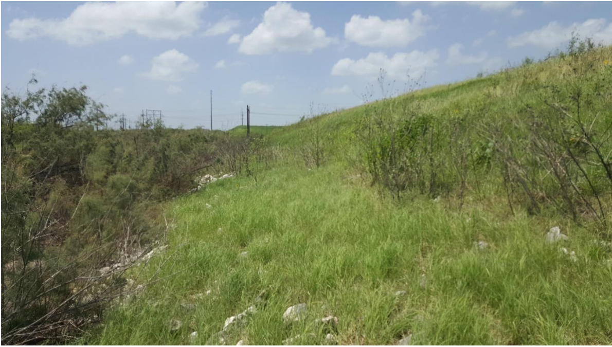
Photo 22 – View looking west at stone riprap and bushes on toe portion of south downstream slope.
