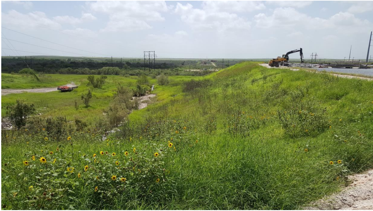
Photo 13 – View looking south along east downstream slope and drainage swale at toe of slope.
