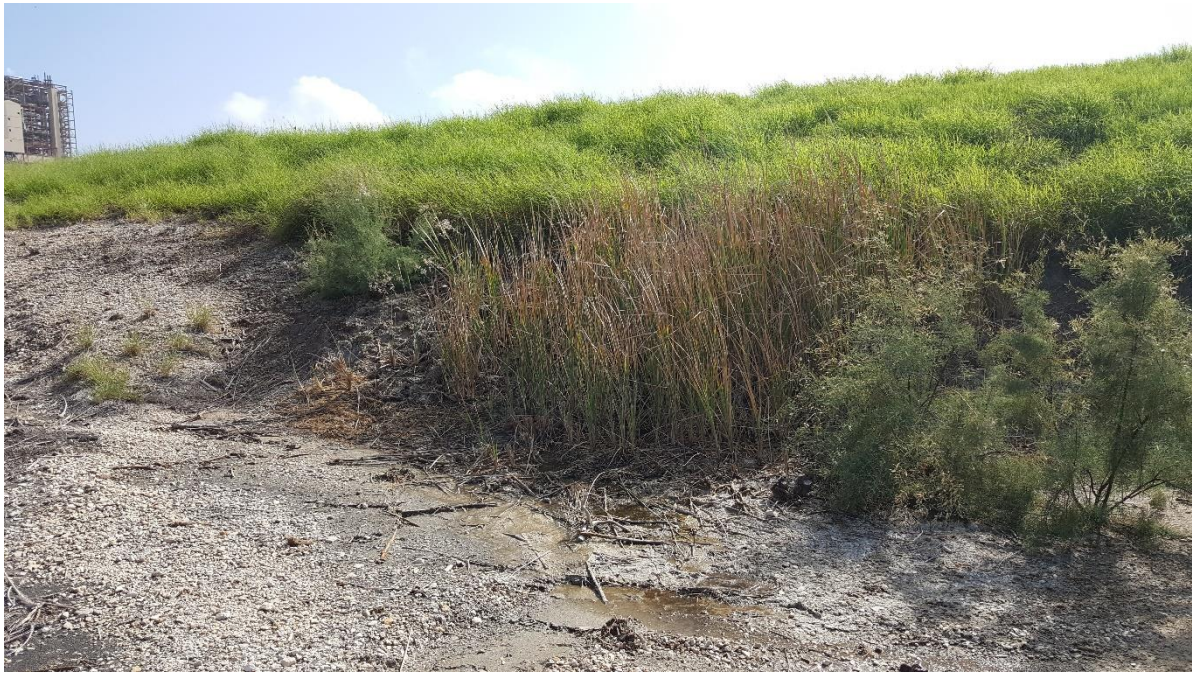
Photo 3 – Close up view of Photo 2 of cattails in steep toe area where seepage is occurring.
