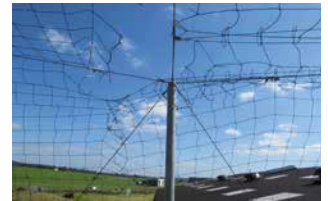
Damaged bird netting
