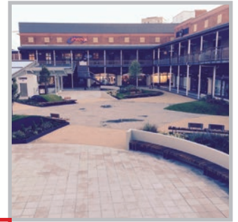
Newton products were used to repair the failed deck waterproofing in the main square of Gunwharf Quays, Portsmouth. Existing paving, grass areas and staircases all had to be removed and reinstated either side of the repair work.
