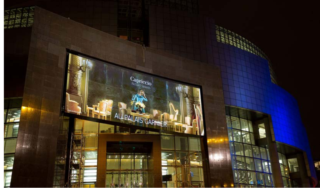
Installation of the giant screen at Place de la Bastille in the autumn of 2015.
