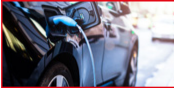
Electric Vehicle Charging Points
