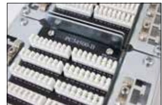
ZTB Internal view showing PCB trays with cable anchor points and shielding clamps
