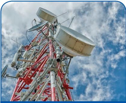
Telecom -Data Infrastructure
