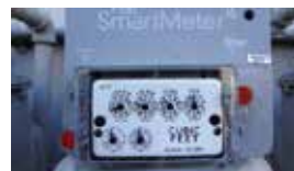
Automated Meter Reading
