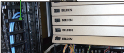
Vertical Manager shown in cabinet
