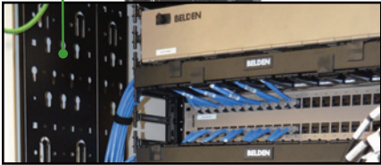
Lacing Panel shown in cabinet
