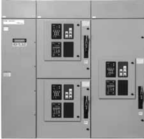
Next Generation AMPGARD Lineup— Front View
