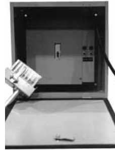
Breaker Test Cabinet
