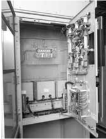
Mark V Field Controller
