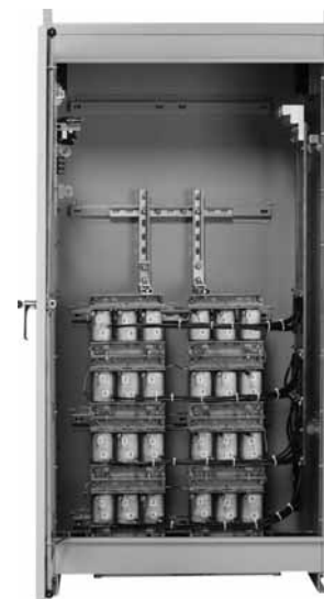
AUTOVAR Filter—Reactor Cabinet
