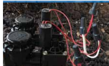
irrigation and sprinkler systems
