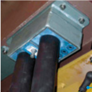
Driver's cabin: The Roxtec S 4x1 is used for mechanical anchorage of cables and to reduce vibration.
