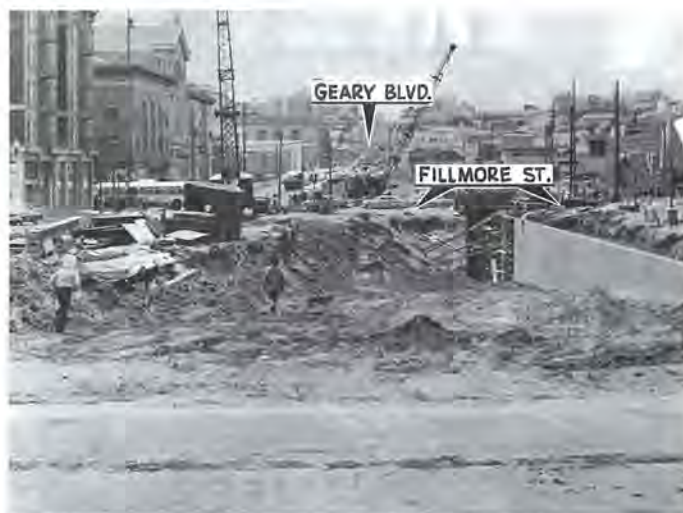
CONSTRUCTION AT GEARY AND FILLMORE STREETS AS PART OF THE WESTERN ADDITION REDEVELOPMENT PROJECT, 1960. PHOTO COURTESY SAN FRANCISCO HISTORY CENTER, SAN FRANCISCO PUBLIC LIBRARY.
