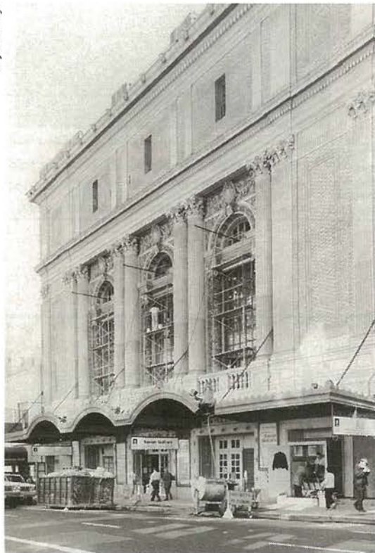
Finishing touches are added to the Geary Theater's historic facade in anticipation of A.C.T.'s January 1996 homecoming celebration.
