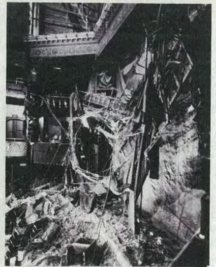
Interior of the Geary Theater, home of American Conservatory Theatre, showing extensive earthquake damage
