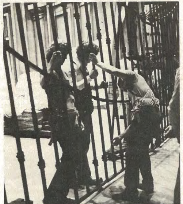
Dan Michalske, Gary Brickley and Nick Bracisco check the iron fence (part of the set seen in the third act) and prepare it for installation on stage.
