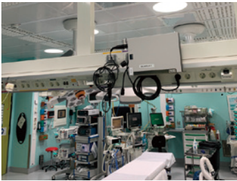
Operating Room with Ceiling-Integrated Filters
