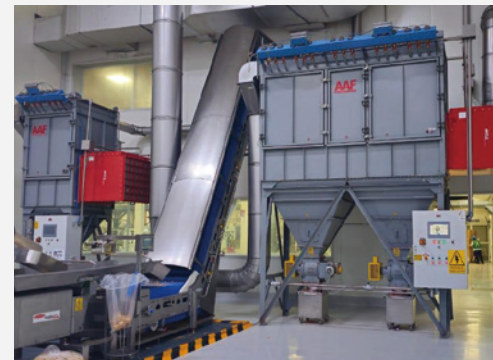
WONDAIR™ at Customer's Plant
