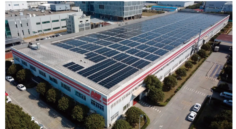
Solar Panels at AAF Suzhou Factory
