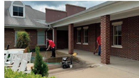
Facility Enhancement Activity
