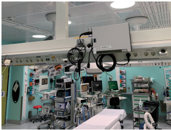
Operating Room with Ceiling-Integrated Filters
