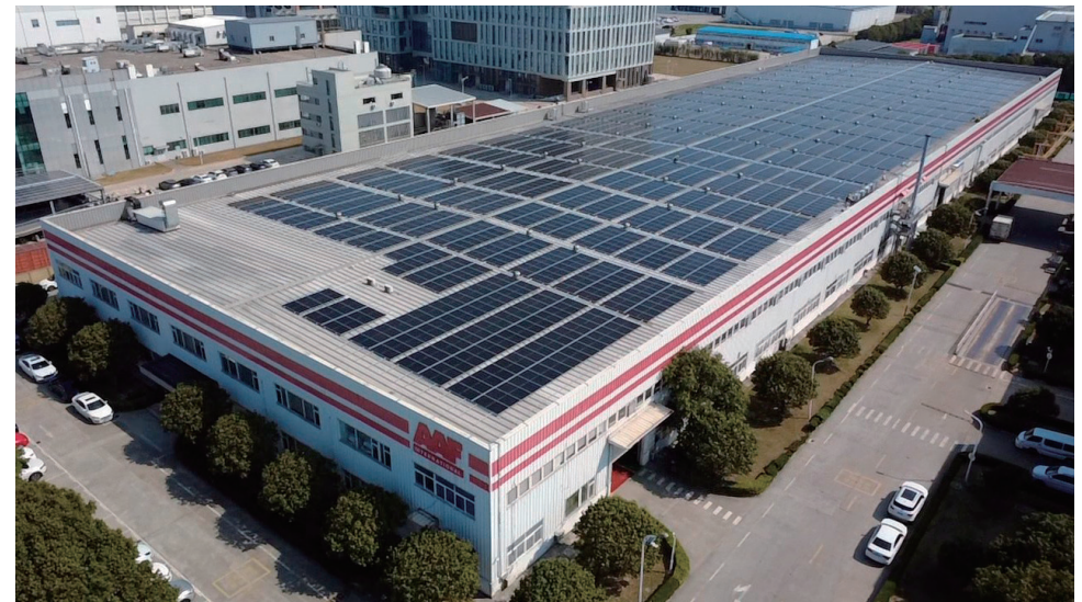
Solar Panels at AAF Suzhou Factory
