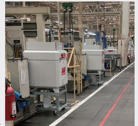
Oil Hunter™ at Customer's Plant
