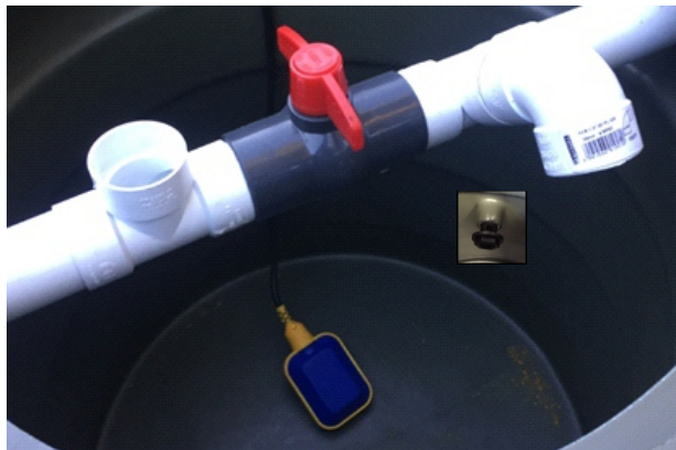
Float switch at the bottom of the tank
