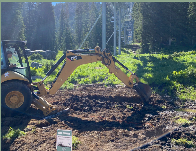
Bend Lot, using an excavator to mimic natural terrain contours and guide water flow | June 2022
