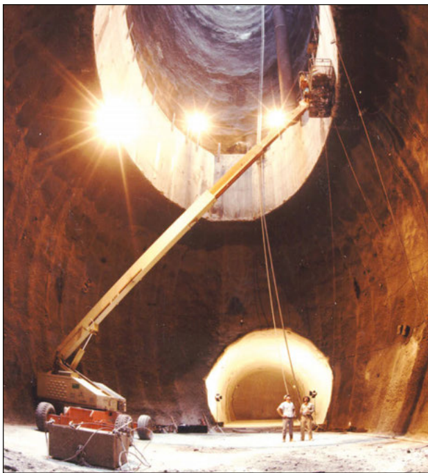
View along the SSC's main ring tunnel, as seen while under construction in early 1993.
