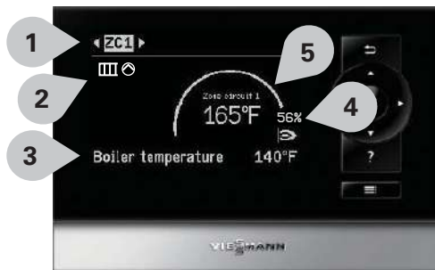
ZC Fixed Setpoint Configured
