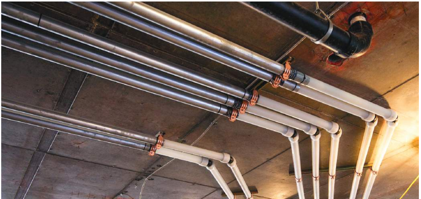
Uponor PEX-a Pipe Support installation at Avalon Bay in Lynwood, Wash.
