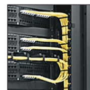
cable management ducts
