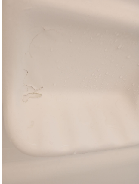
Sample Chipped paint in various areas of the Bathroom
