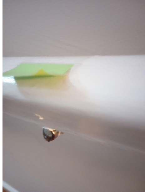
Sample Chipped paint on banister in the hallway near living room
