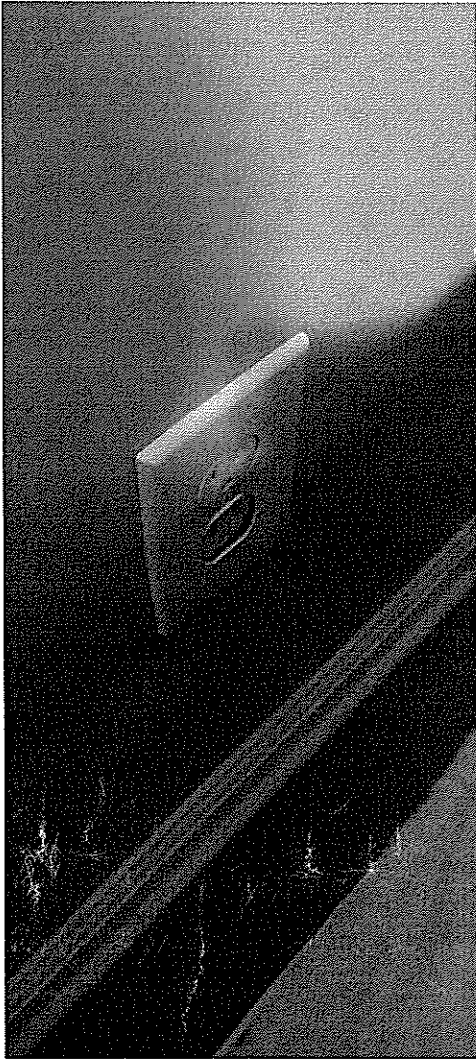
Socket needs to be fixed
