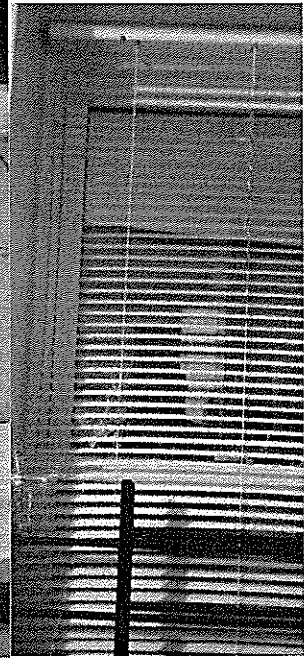
blind closer missing
