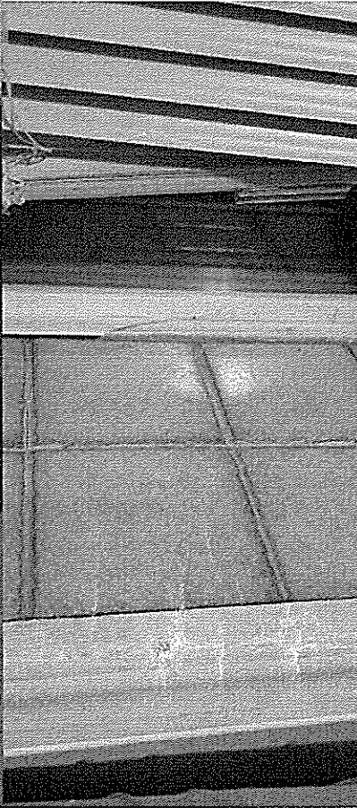
piece of the window seal is missing
