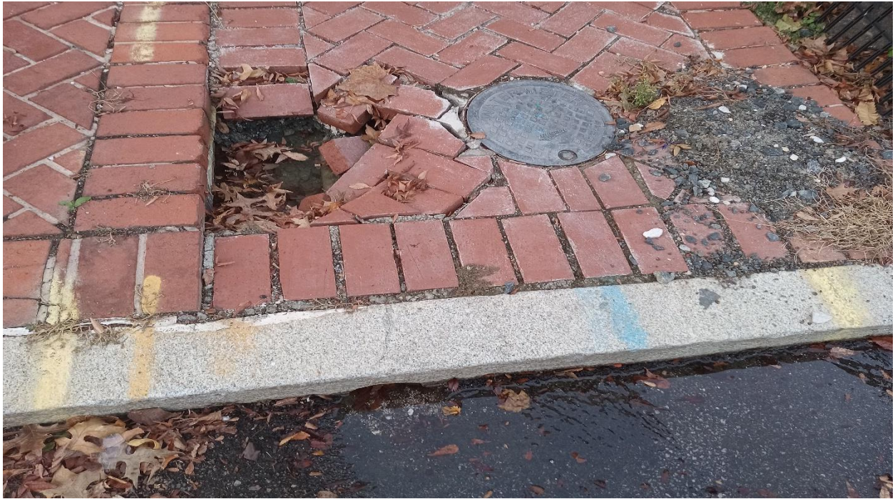
Photo 3: Another picture of the broken sidewalk with water in the vault of the water meter at 711 Druid Hill Avenue. You can also see water running out of the drainage pipe of my entrance way.
