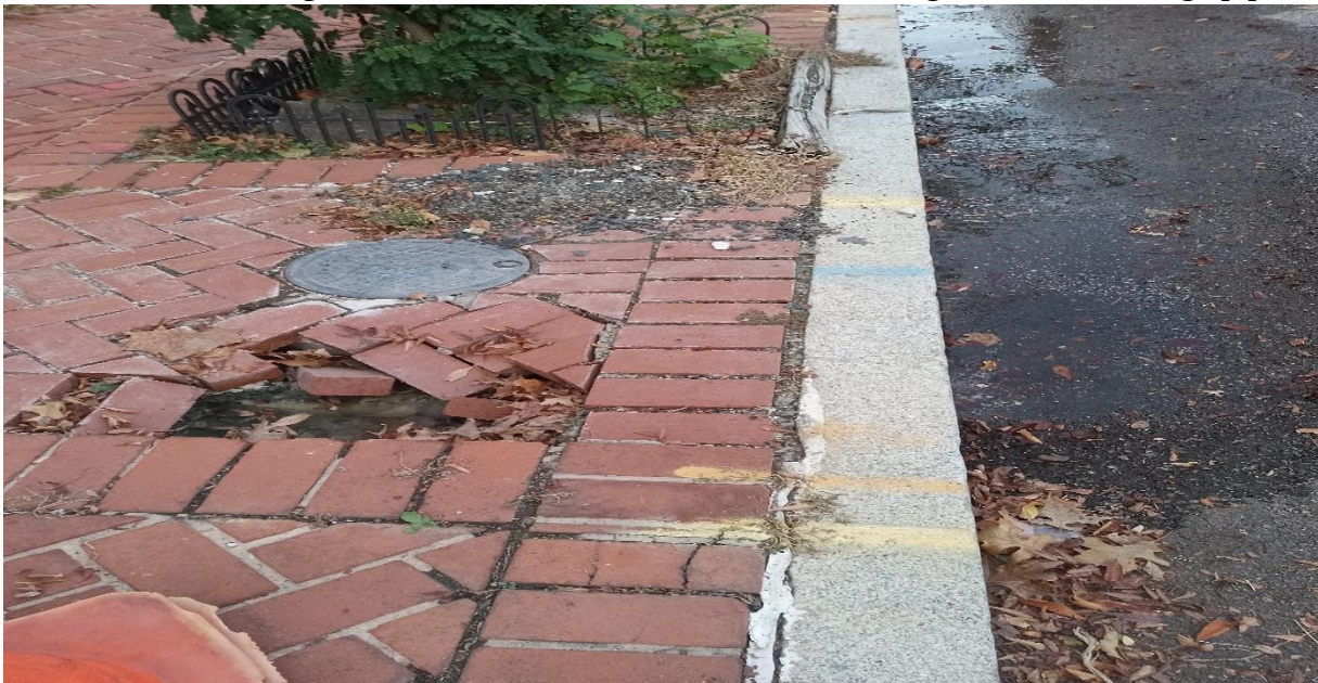
Photo 4: Another angle of the broken sidewalk with water running out of the drainage pipe.
