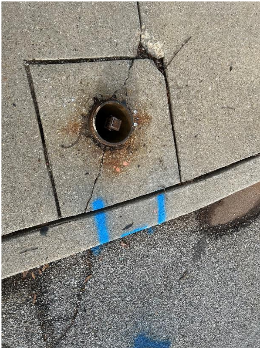
The Fire Hydrant was knocked out. It is located on the intersection of Liberty Rd and Resource Drive in Randallstown.
