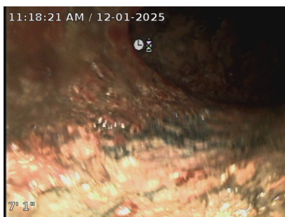
Slight right bend. Connection to additional indoor plumbing.
