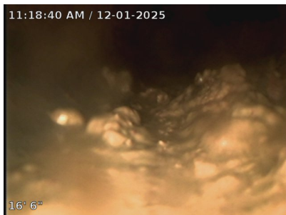
Minor sludge in cast-iron portion.
