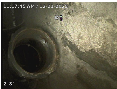
Start of video. Entry point PVC cleanout in basement floor near front of house.
