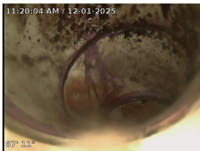
Downward bend just before snake line in front yard.
