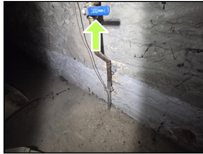
The main water shutoff valve.
