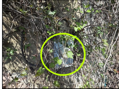
The electric meter located at the rear of the property in the basement.
