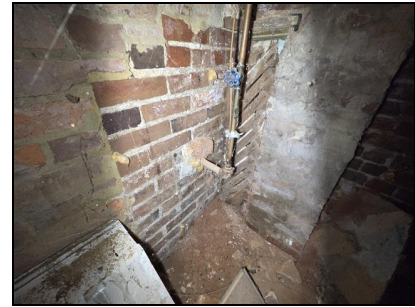
The main water line and shutoff valve
